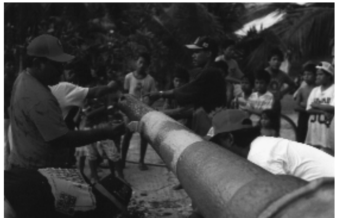
Two different primers with corrosion inhibiting pigments were used to test their effectiveness in the severe tropical marine climate.
